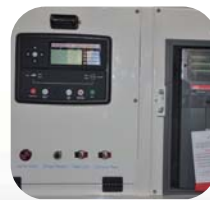
Control Panel & MCB
